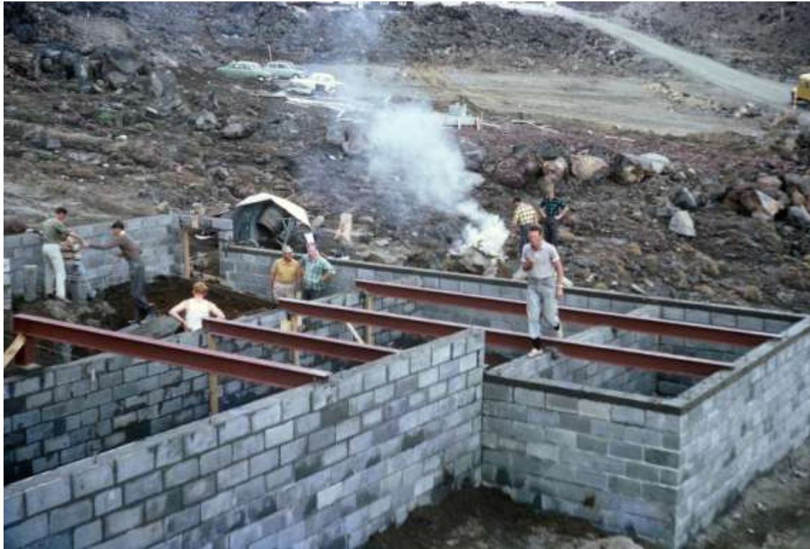
Figure 2 Block work progressing. The water tank is below the central steel beams. 19 April 1965
